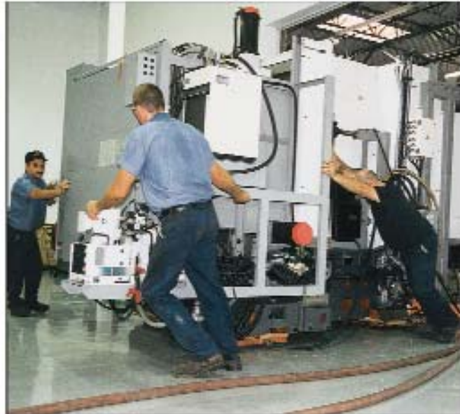
Maxiforce Lift Bags used to position "Air Casters" for machine tool positioning.
